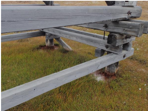
Line 6, Bukk 27 (pictures 27_5 and 27_7) – changes in vegetation and depressions around foundations, spin-off effect – ponding of water
